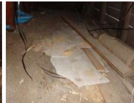
Above: Cement sheet debris below floor.
