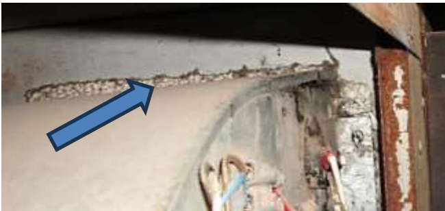
Above: Asbestos rope gasket between equipment parts.
